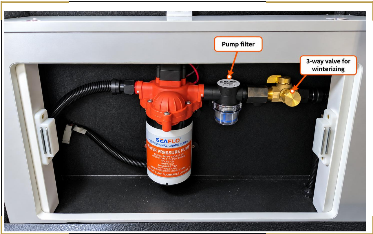
WATER PUMP FILTER AND PUMP WINTERIZATION VAVLE LOCATION
