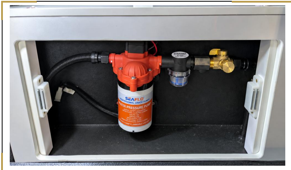
WATER PUMP LOCATION
